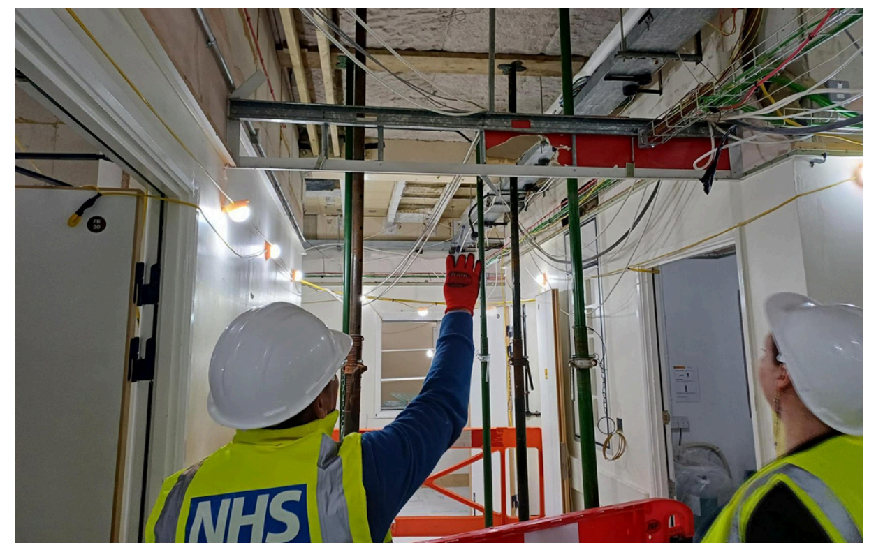
RAAC in theatres at Frimley Park Hospital
